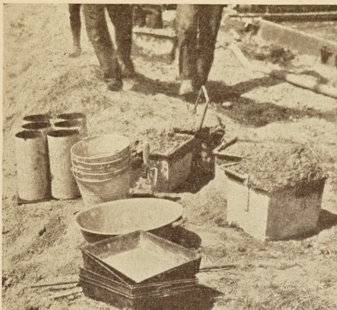
REMOVING SAMPLE BUCKETS AND BEAMS FROM THE SUBGRADE TO THE BERM OF THE ROAD, WHERE ANALYSIS WAS MADE OF THE FIVE PARTS OF THE BATCH FOR THE EXACT AMOUNT OF GRAVEL, SAND, CEMENT, AND WATER.
